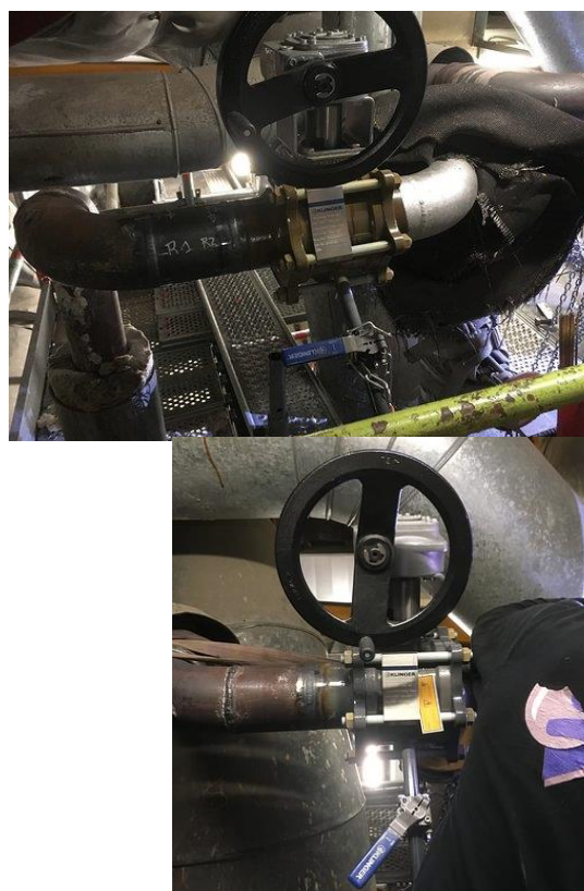
KHA-SL DBB installed to make the steam network safer.
